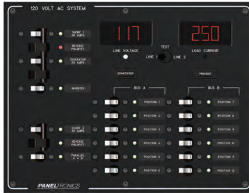
3309 13.75" W x 10.5" H x 3.5" D AC 12 Position with Dual Shore/Generator/Inverter Mains and Meters
